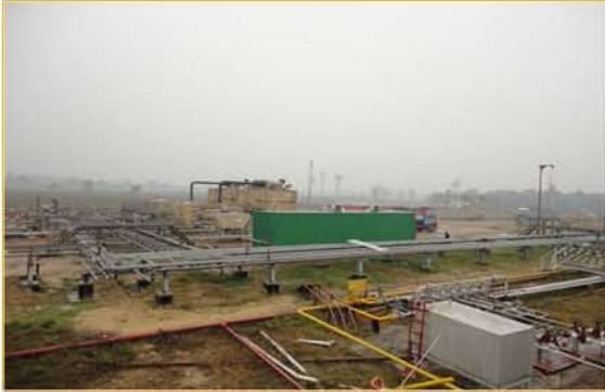
Gas Compression Facilities
